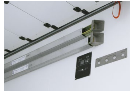
When not in use, the load shift protection beams are secured at the side on the wall.
